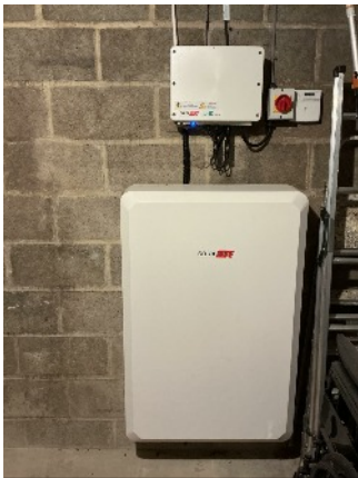
Denise's solar inverter and battery, in her garage
